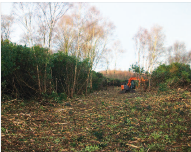
Above: Dense rhododendron clearance during Phase 1 on Thorne Moor. A coarser finish was left in order to retain some mosses and lichen and provide increased cover for ground nesting birds.
